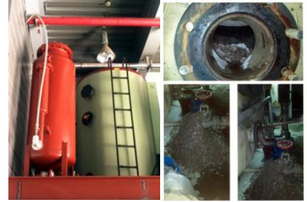
(3) Dyeing factory in Korea To scale the boiler they have.
